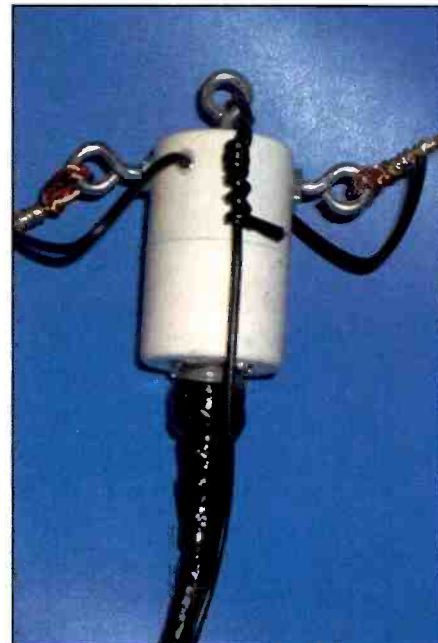
Photo C. The coax connection at the center insulator should be properly weather-sealed to avoid water damage. Note how the coax messenger coax is tied off to the center insulator support eye ring.
